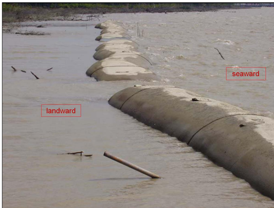
Figure 5.9: Sand-filled geotextile tubes used in Tanjung Piai, Johor, Malaysia to reduce wave energy on mangrove shoreline. Note that the area seaward of the tube is very turbulent while the area landward is calmer, which will enhance sedimentation of mud on the landward area (after Ghazali, 2005).
