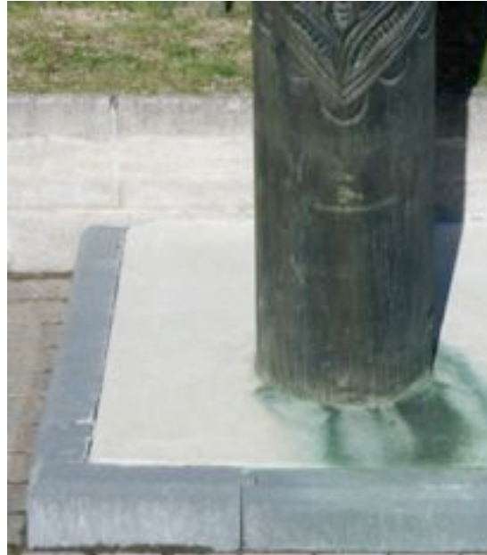
Figure 1.21 Greenish leachate staining the concrete in front of a CCA-treated pole.
