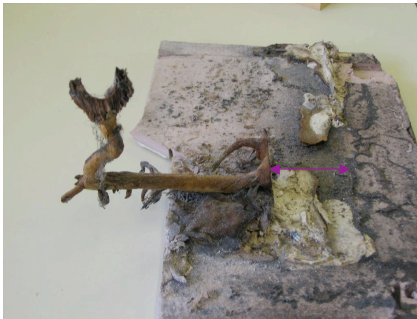
Figure 2.2 Fungal fruiting body Lentinus squamosus detected behind monolithic cladding material. Note: Magenta arrowheads indicating the original positioning of the wall framing (Courtesy of Beagle Consultancy Ltd., Rotorua, NZ).
