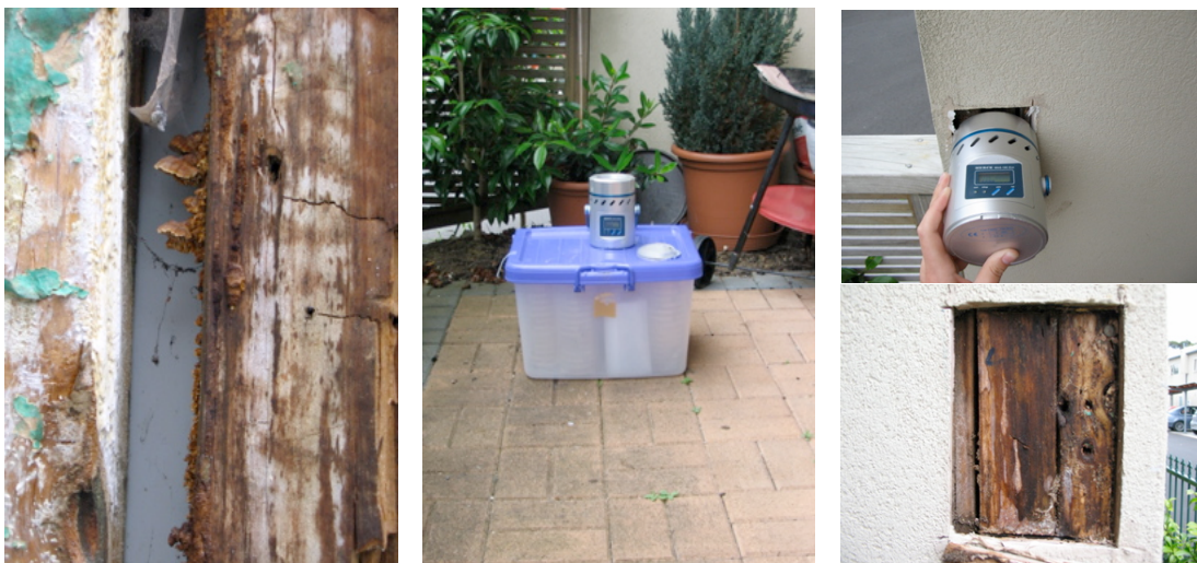
Figure 4.1 Left : Gloeophyllum sepiarium fruiting body on framing stud and associated white mycelium. Centre : outside sampling ground level. Right, upper : sampling within wall cavity. Right, lower : decayed and damp wall framing.
