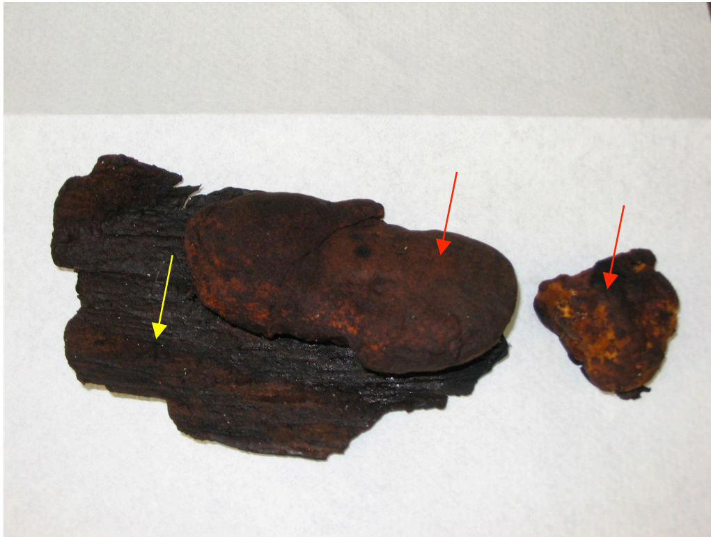
Figure 2.5 “Dark” fungal fruiting body samples (red arrows) without any prominent identification features; already detached from the framing timber but still connected with a thick and tough fungal mycelium mat (yellow arrow) (Courtesy of Beagle Consultancy Ltd., Rotorua, NZ).
