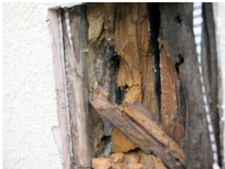
Figure 1.16 Corner wall stud heavily degraded and exploited for nutrients by decay fungi.
