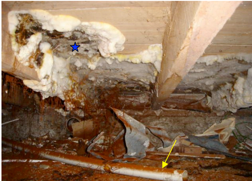
Figure 2.3 Fungal fruiting body Serpula lacrymans development under house floorboards (blue star); Red 'dust' on the ground and on various building materials are reproductive spores produced by this fungus (yellow arrow) (Courtesy of AA House Checks Ltd., Christchurch, NZ).
