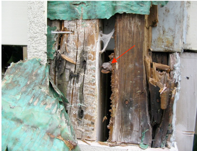
Figure 2.1 Fungal fruiting body Gloeophyllum sepiarium growing between two vertical studs (red arrow); detected after exterior wall cladding material was removed.
