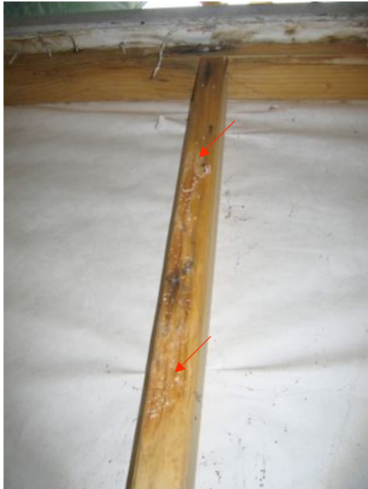
Figure 1.14 P. radiata wall stud showing early signs of decay establishment on the surface, indicated through formation of white mycelium (arrows). Source: Prendos Ltd., Auckland, NZ (2007).
