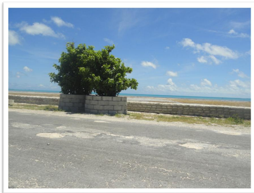
Figure 2.1 Sea wall at Nanikai to protect coastal erosion
