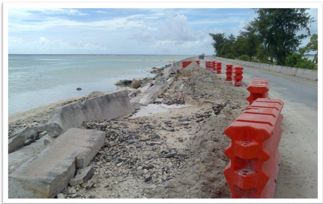
Figure 6.1 Damage of Dai Nippon Causeway by King Tide 2014
