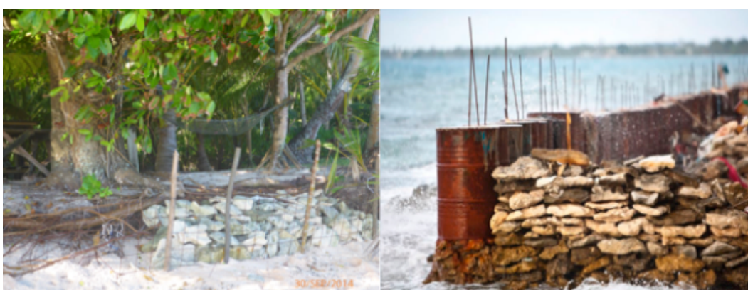
Figure A1.2: Small-scale seawalls in Tuvalu. Source: Author's own photo (left photo is a place in Nui) and courtesy of Apinelu Tili (right photo is a place in Funafuti).
