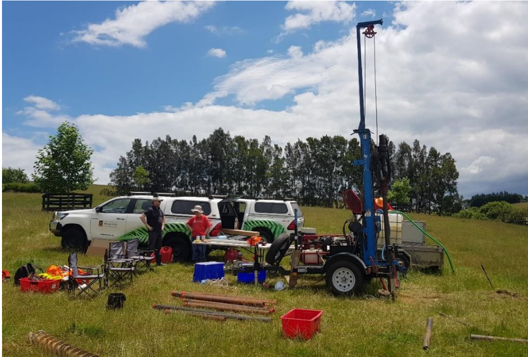
Figure 3.2: The drill rig and processing set up for DH1 in Karaka. The drill rig is operating on a low point within the tuff ring with water tanks and processing tables behind it.
