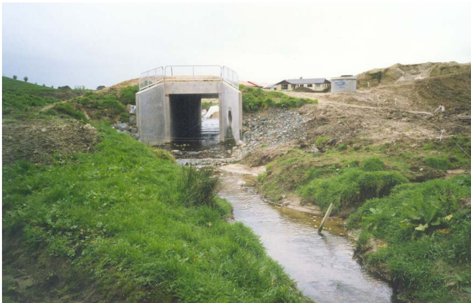
Figure 4. The 3m by 3m concrete culvert under the proposed Magellan Rise (photo: Brendan Hicks, 21 September 2001).
