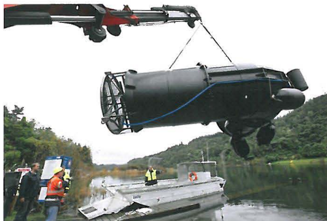
Figure 3. A section of a destratification device prior to installation in Lake Rotoehu. Image: Andy Bruere
