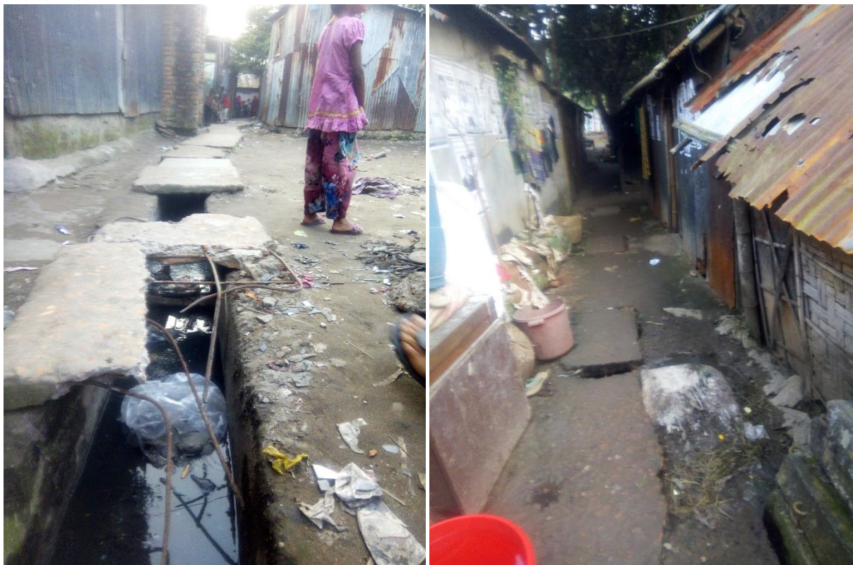
Figure 5.7 and 5.8: Broken drains in the Beguntila slum Source: Field survey (2018)
