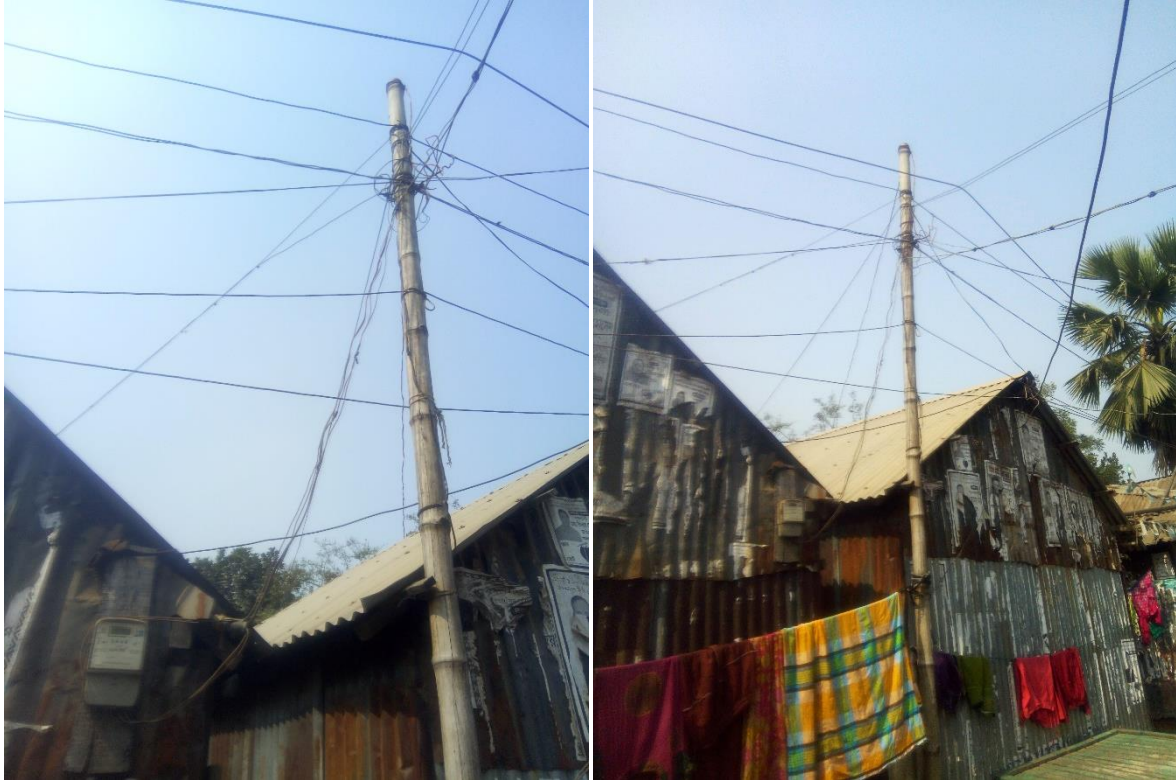
Figure 5.9 and 5.10: Electric wires hanging on light bamboo poles over tin-shed house Source: Field survey (2018)
