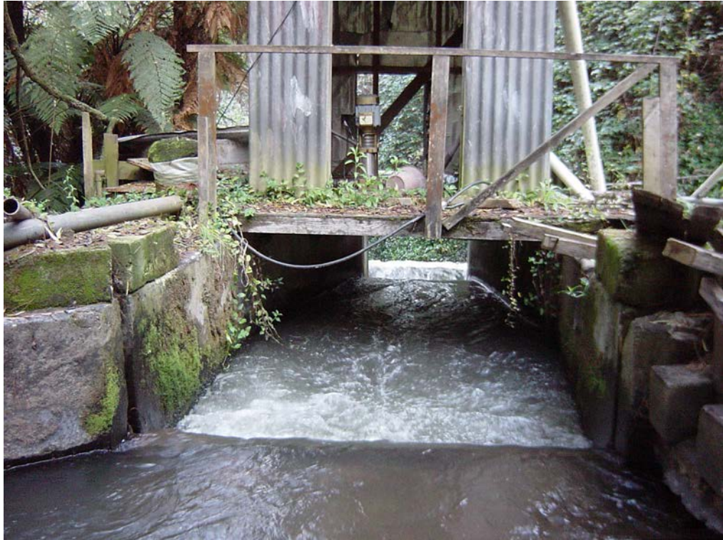
Figure 143. Downstream view towards the flume structure at Site 15.2 in the Wairakei Stream.
