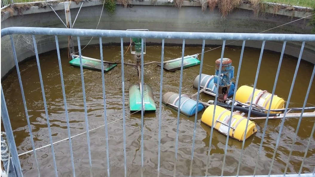
Figure A-3: Stirred dairy effluent sump
