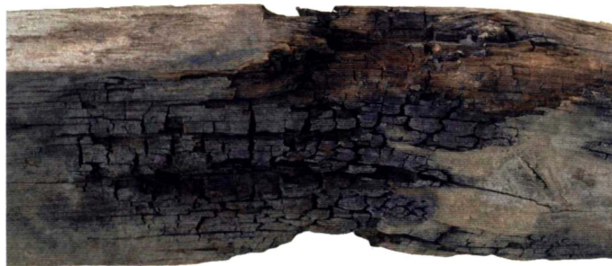
Figure 1.2: Damage caused by a brown rot decay fungus on untreated timber (Photo courtesy of Forest Research).
