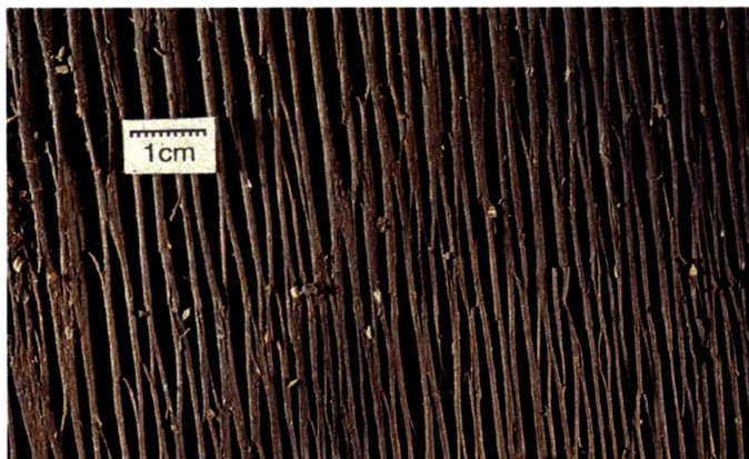
Figure 1.4: Damage caused by a soft rot fungus on untreated timber (Photo courtesy of Forest Research).
