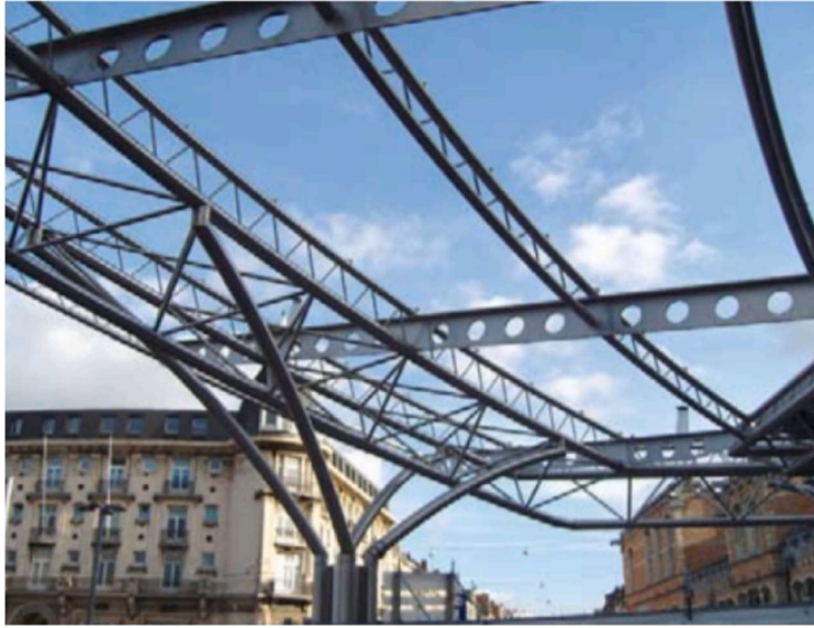
Figure 1.1: Structural stainless steel at Gent Sint Pieters railway station in Belgium. Photo: Patrick Lints [41,11]
