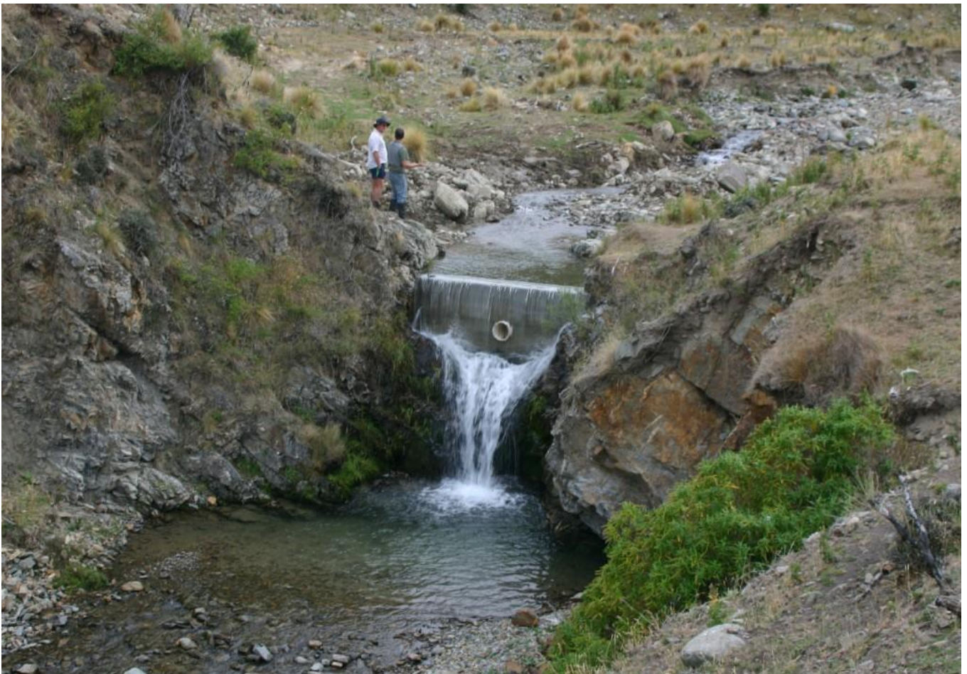
Figure 3.5 Swinburn Creek barrier in Central Otago. A built barrier has been installed onto a natural waterfall to protect Central Otago roundhead galaxiid populations, after brown trout gained access upstream when stream conditions changed (Source: Department of Conservation, 2018).
