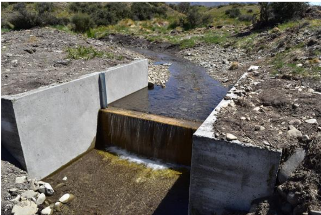
Figure 3.7 Built barrier installed in Cabbage Tree Gully, South Canterbury. The barrier was built to prevent trout accessing a key lowland longjaw galaxias population, Canterbury (Source: Department of Conservation, 2018).
