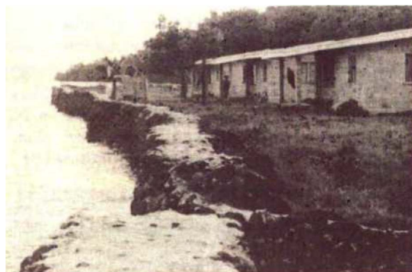
Figure 24 Stone and cement sea wall protects new houses at Rukua (1981) (Source: Rajotte & Bigay 1981:14)
