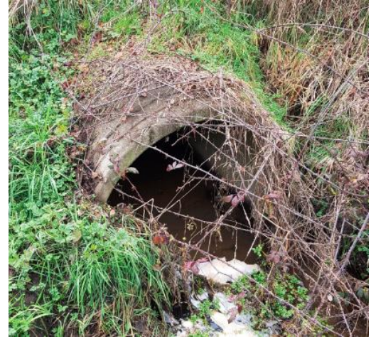
Figure A.14. Pipe draining detention bund at OK3
