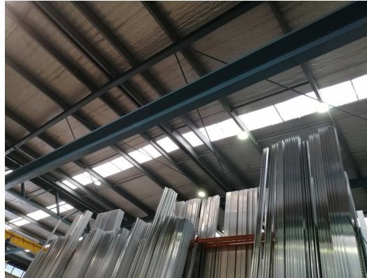
FIGURE 3.1: Ceiling and lighting above extrusions in the APL warehouse.
