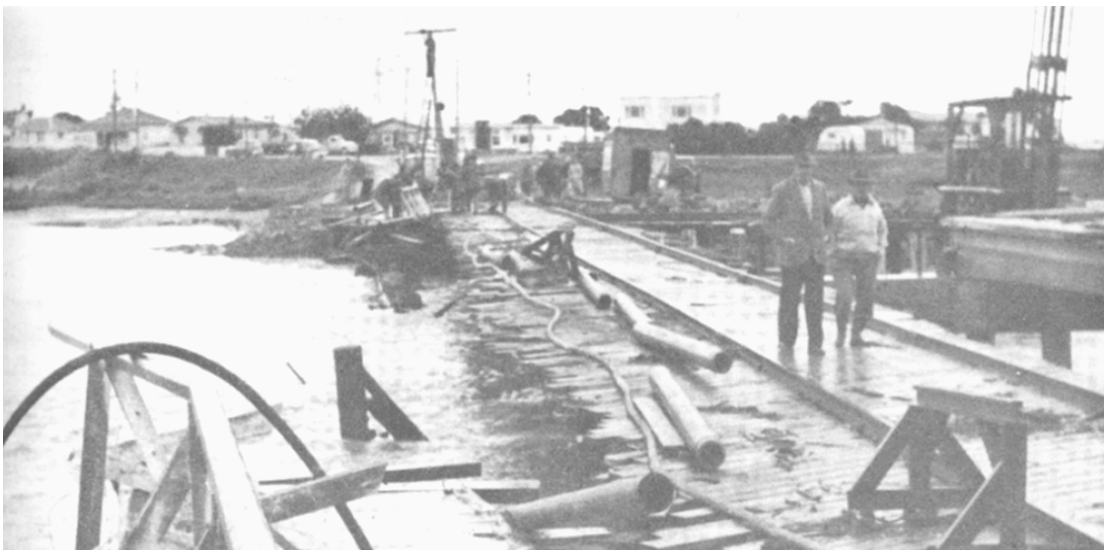
Figure 2.2: Damage to the Ahuriri footbridge in Napier following the 1960 Chilean tsunami. (Source: The Daily Telegraph, 1960).
