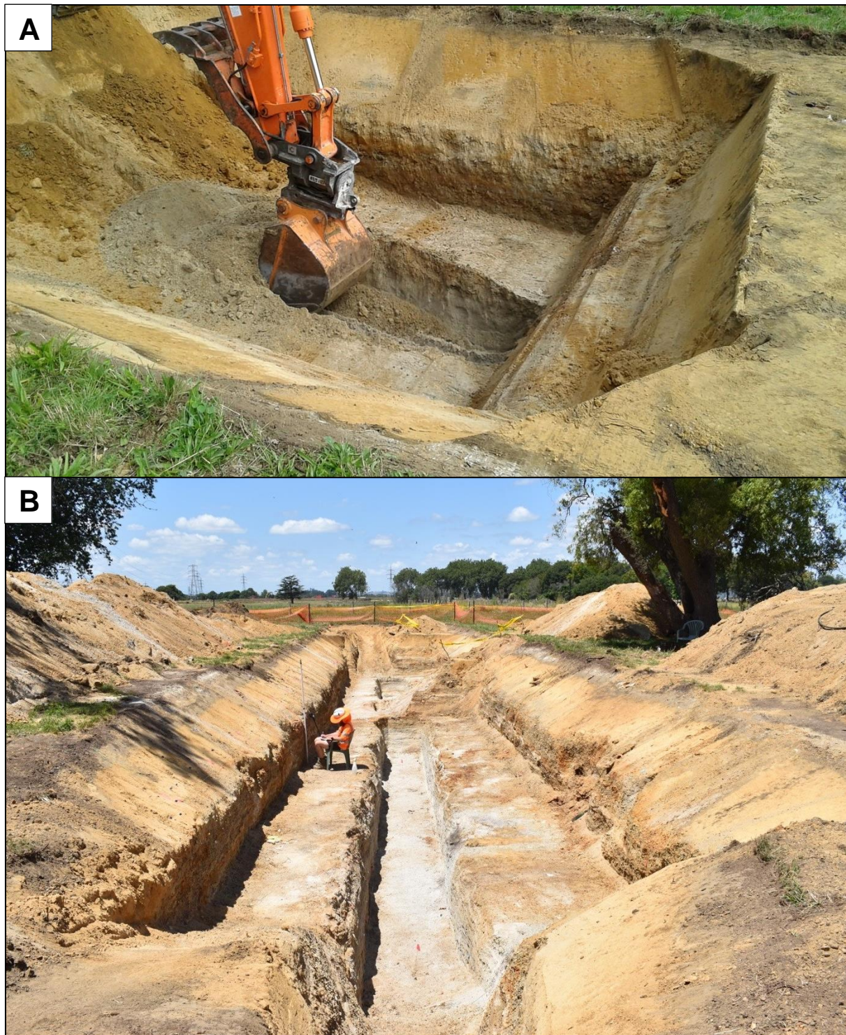
Figure 2.6. Photographs of trench excavation showing; (A) first section being excavated, illustrating the method of cutting a complete profile in increments rather than progressively deepening the complete trench length; (B) view along the completed trench towards the east, showing the full as-cut profile. The north wall to the left of image was comprehensively logged while the south wall was considered less suitable due to the level of human disturbance.
