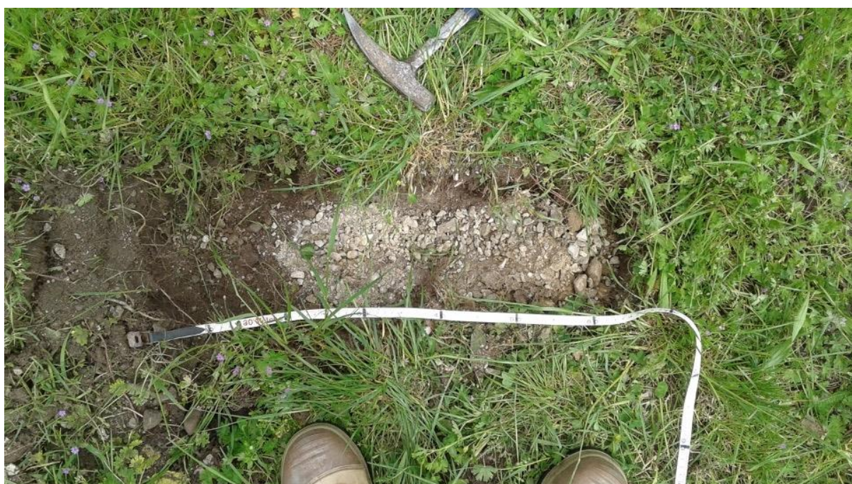
Figure 4.28. Photograph of hand cleared section of topsoil, confirming presence of limestone and concrete chips from old driveway.
