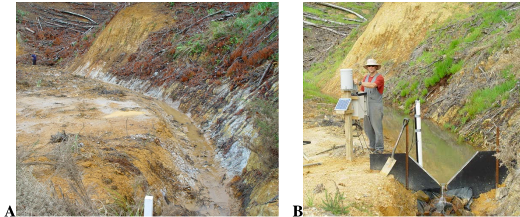
Figure 8.5. A) The EX-H6 subcatchment before the installation of monitoring equipment. A drain has been cut and to the left is the edge of the log landing and to the right of the drain is a formed batter. B) The eventual location of the temporary plywood weir and monitoring equipment.
