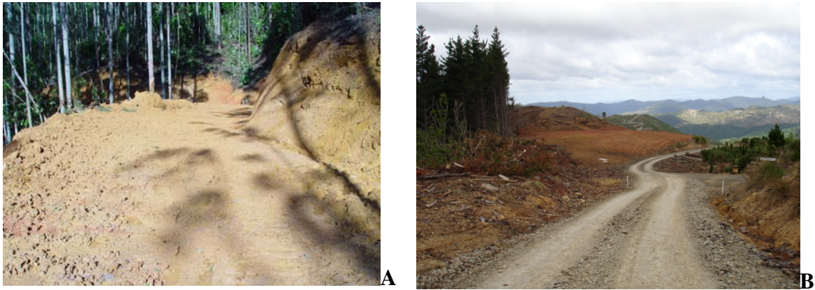
Figure 2.9. A) Newly constructed access road and batters into a logging compartment; B) newly formed log landing in the background and a metal sealed access road.
