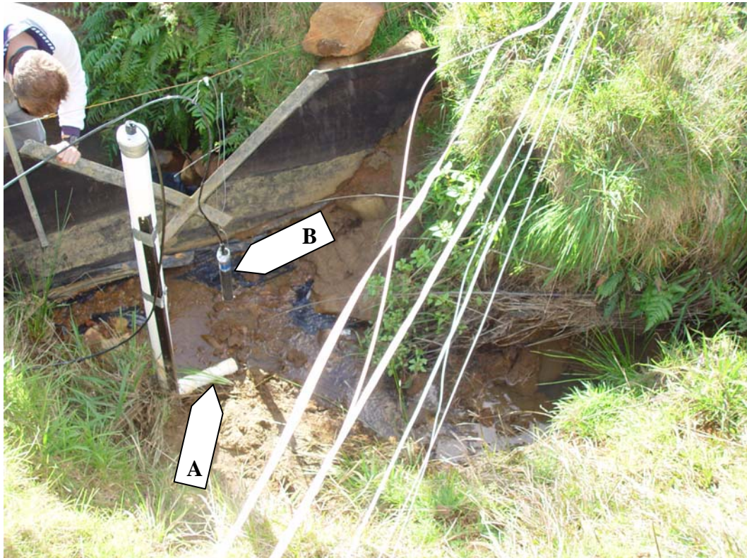
Figure 8.12. Monitoring equipment installed at the AG-P site emptied of water after weir failure (note water height stain on the weir face). A) The original mounting for the turbidity probe at right angles to the stream flow. The original mounting was around 30 cm above the stream bed but coarse material has deposited behind the weir. B) The suspension deployment of the turbidity probe upstream of the V-notch weir.
