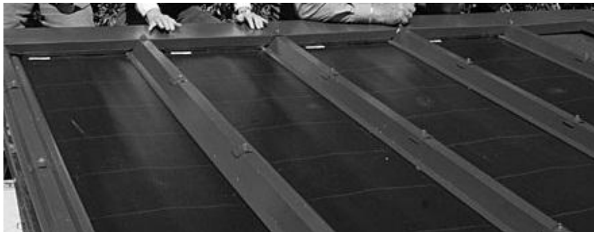
Figure 24 - Solar rib installation completed in March 2010 on Dumpling Hut on the Milford Track
