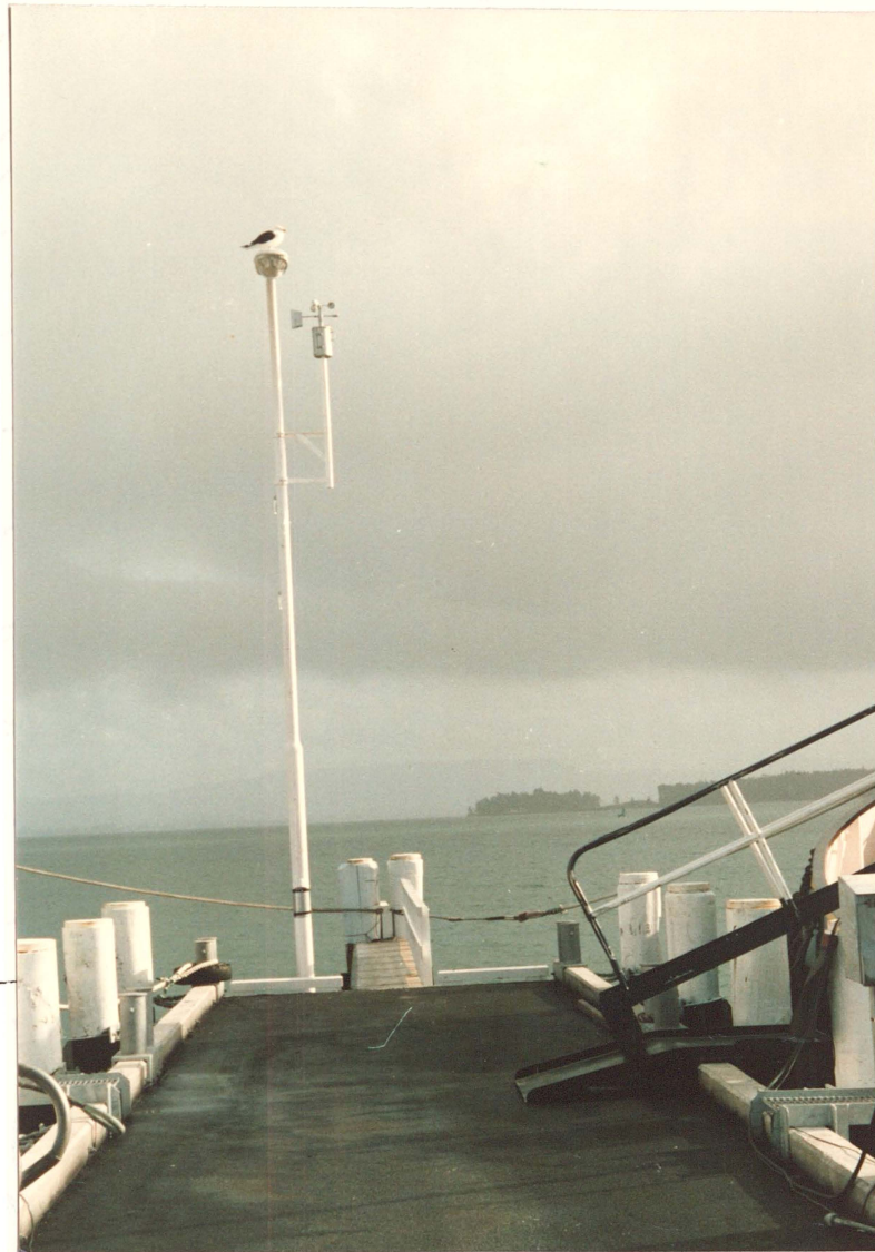
Plate 4.1 - Woelfle Anemometer installation on the southern BOPHB Tug Berth. A fork lift provided access to the anemometer for servicing.
