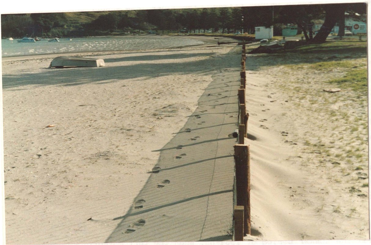
Plate 7.3 - Polypropylene break fencing constructed adjacent to the renourished beach, May 1984. This fence effectively stopped the onshore movement of fine sand from the back beach area. The immediate area surrounding the fence was subsequently sprayed with grass seed, producing a reasonably continuous turf out to the position of the aluminium dinghy.
