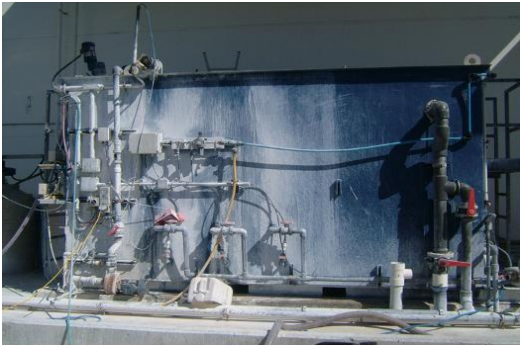
Figure 3. 2 CPS unit for trade waste treatment at Finex
