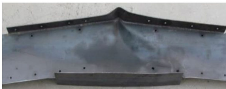
Figure 2-15 Buckling failure of apex brackets after Öztürk and Pul (2015)
