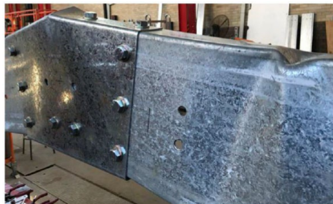
Figure 2-19 Local buckling of flange-web junction in the apex joint test after Rinchen and Rasmussen (2019b)
