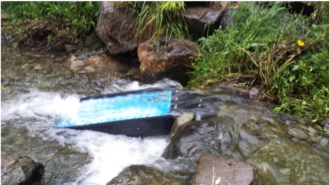
Figure 5.1: A 'Half ramp' which has been cut down to 1.2 m in order to fit in the short plunge pool of the Brook Stream, Nelson. Note blue colouration of plastic panels from early manufacturing runs. Panels are now black.
