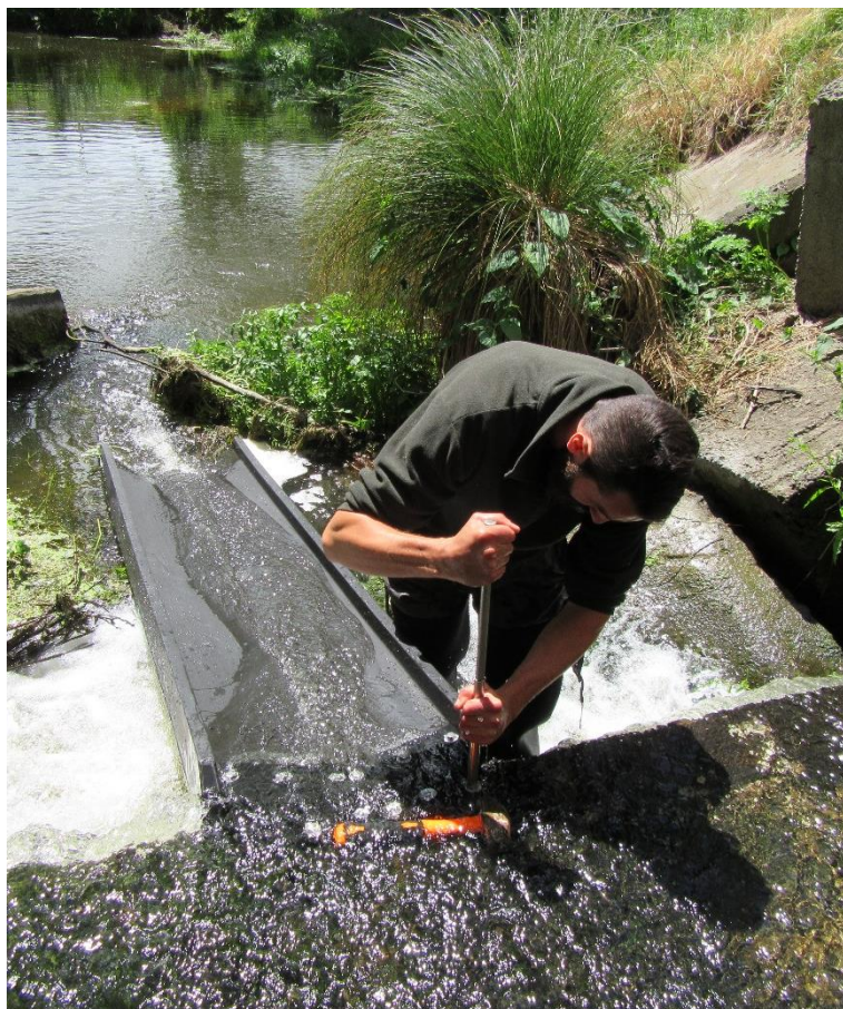
Figure 5.2: The author using a slide punch to hammer in mushroom spikes during installation of the Awanui ramp. Note the absence of textured panels at this stage of the installation.
