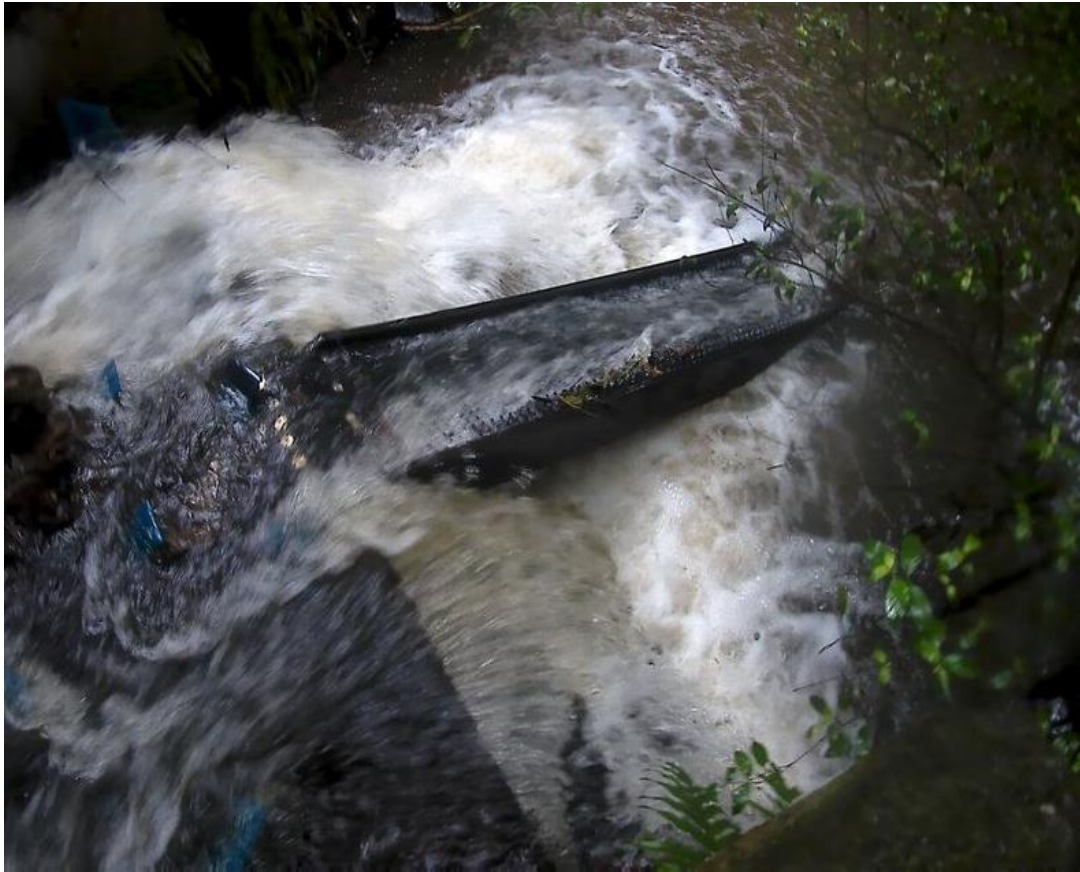
Figure 5.5: Floating fish ramp in the Kakahotoa Stream, Matahina catchment, Edgumbe. Photo taken post Cyclone Debbie. Note flexible baffles directly above the ramp. Photo credit: Kelly Hughes, ATS Environmental.
