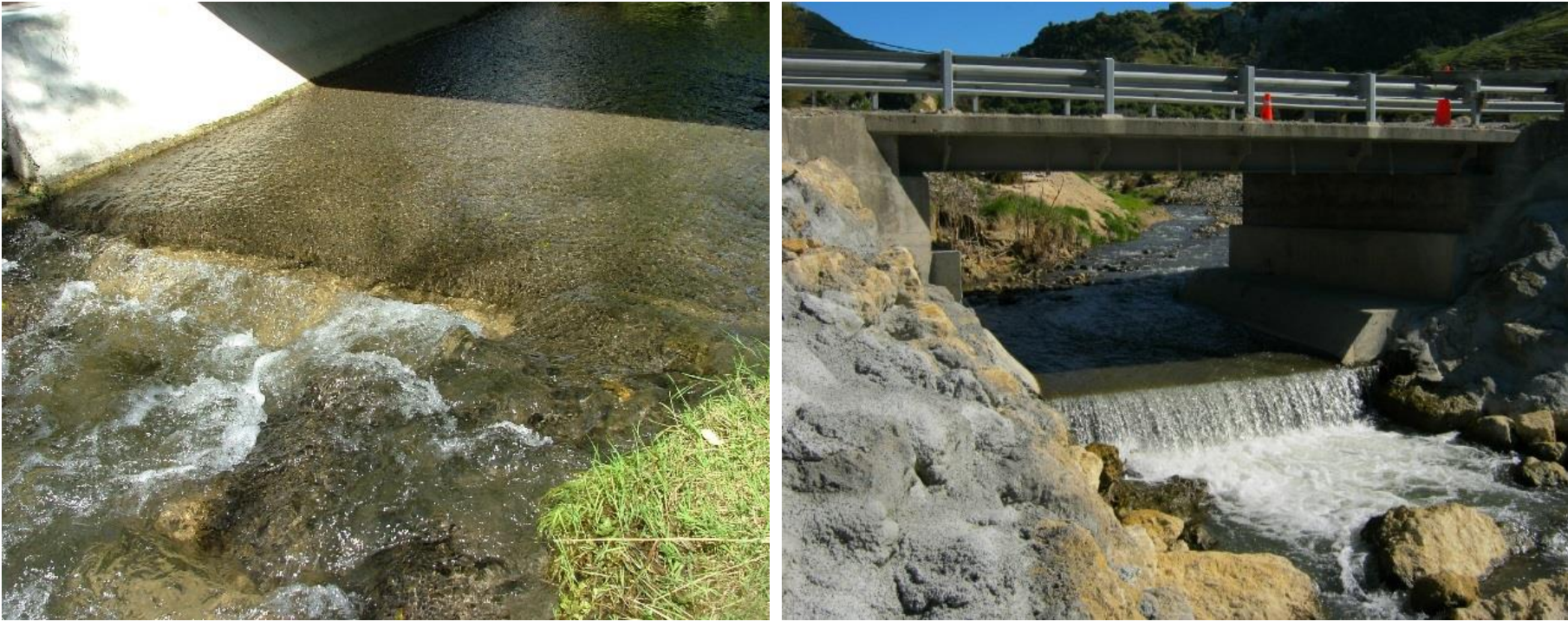
Figure 2.6: Pictures showing degree of perching on the downstream end of concrete pad in Waingongoro Stream, pre-flood event (left) and post-flood event (right).
