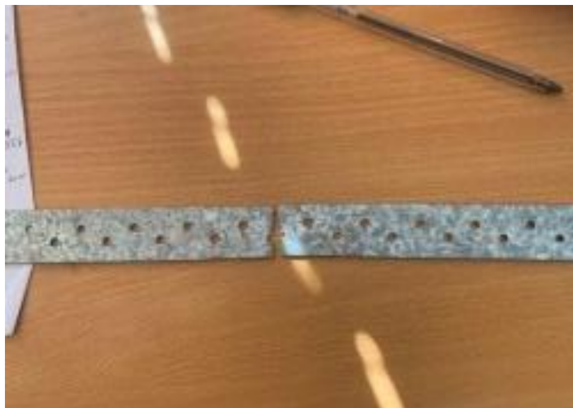
Figure 34-The snapped 25mm steel reinforcement strap
