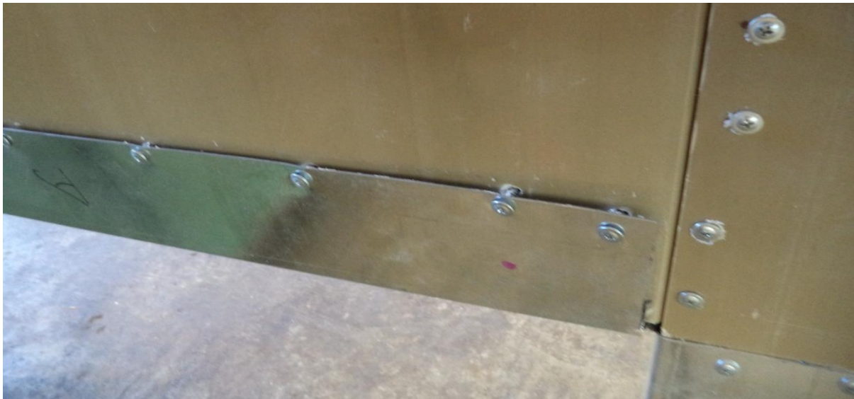
Figure 55-The screws fixing the bottom channel were pulled out
