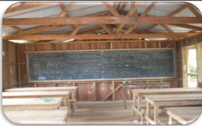
Figure 5 Incomplete classroom block
