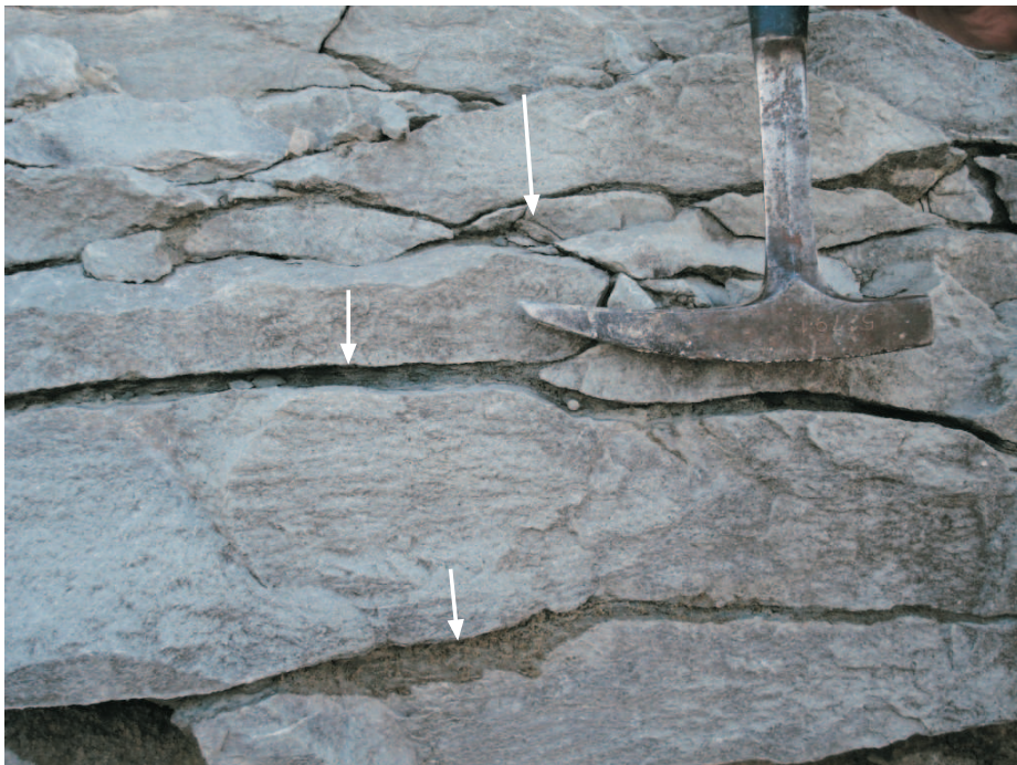
Figure 3.7 Thick discrete dissolution seams (white arrows) in the Aglime limestone unit that have preferentially weathered back to produce a flaggy limestone, northern face, on road to drying plant.
