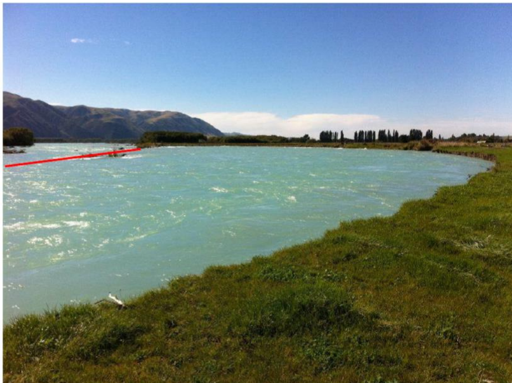
Figure 7.40 South Bank of Waitaki River, near Duntroon, looking north-east, 10 March 2011, showing damage on riverbanks as shown by the red line. Approximately five hectares of productive land was lost to the River during the event. An intake and headrace structures were also destroyed during sustained high flows [145].
