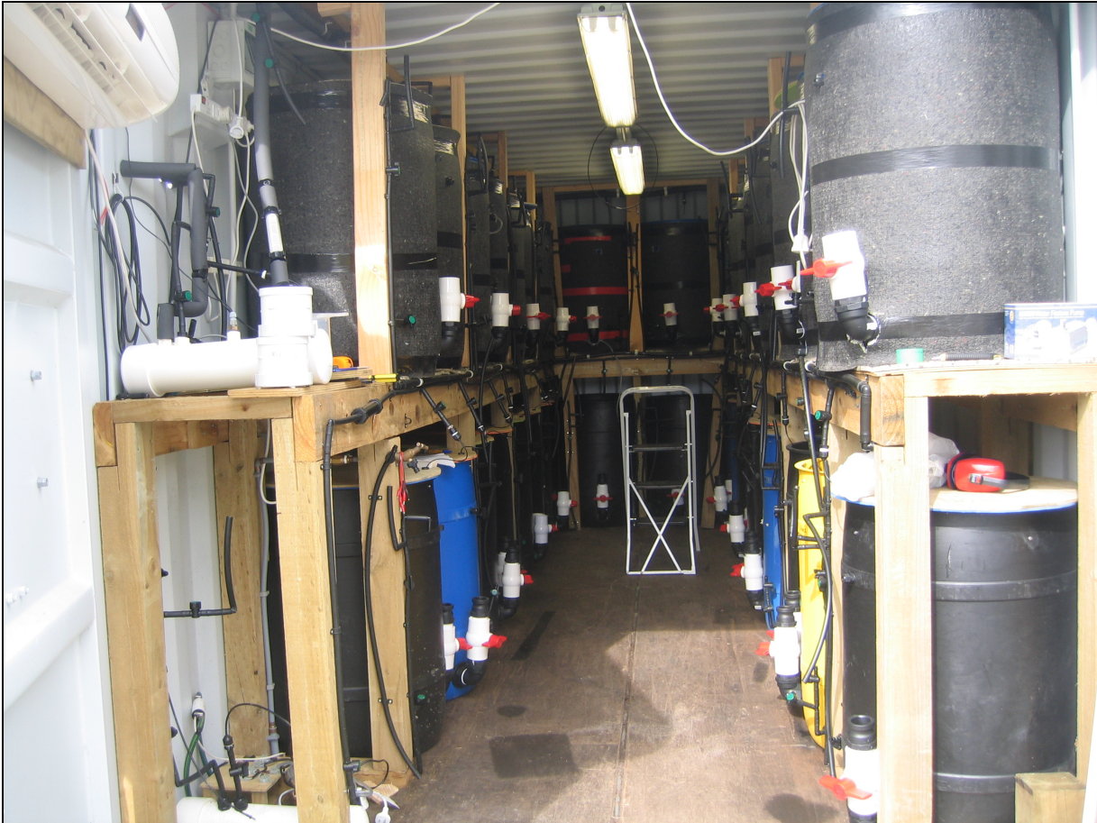
Figure 3.1 Photograph of barrel trial. The photograph shows the 0.2 m 3 barrels housed within the 7.5 m long shipping container. The unheated 14°C barrels are located on the floor of the container. The heated 23.5°C barrels with thermal lining are located on the wooden shelving. The heat pump that maintained temperature in the container is at the top right hand corner of the photo. The 200 mm diameter PVC tube mixing manifolds are on the left hand side of the entry to the shipping container. The manifolds were used to mix the dosed KNO 3 solution with the influent water before being piped to the barrels.
