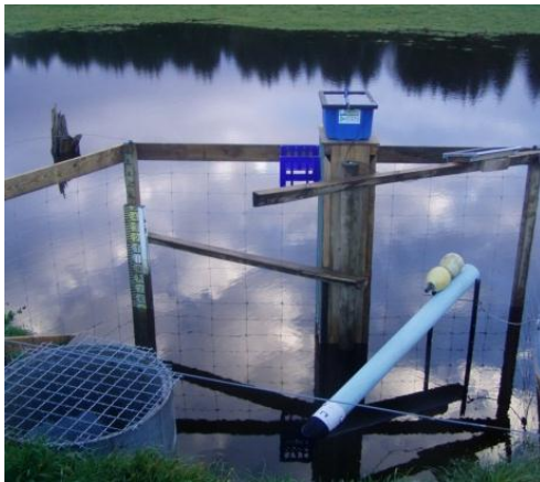
Figure 2.10: Water level recording system housed in the vertical structure with the blue box on top, powered by a solar panel (top right). Hauraki DB, July 2012.
