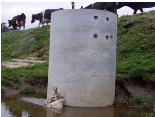
Figure 2.14: The riser at Awahou DB had an outlet at the base, which was plugged by a sand bag that was pulled using an attached rope.
