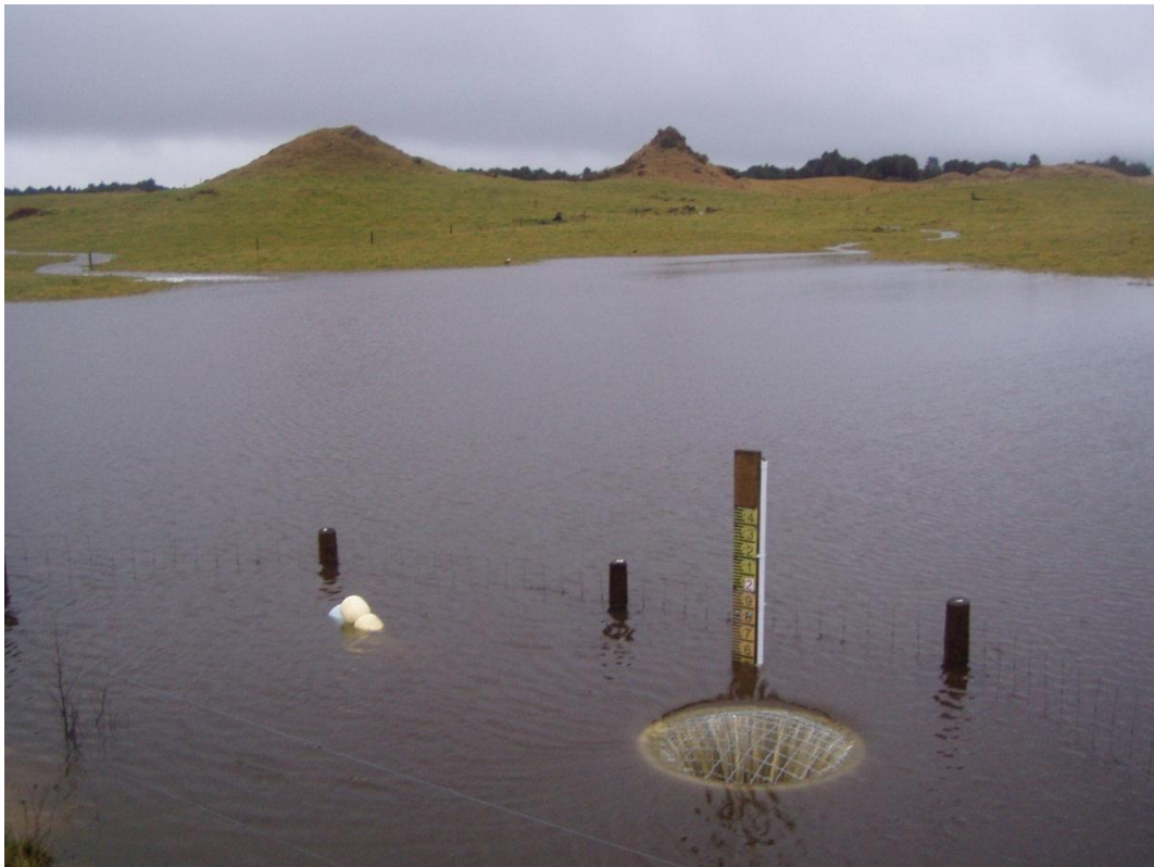
Figure 1.7: A full detainment bund in the upper Waiteti Stream catchment in 2012.Ponded water exits down the top of a concrete riser (outlet #2) when storage capacity has been met.
