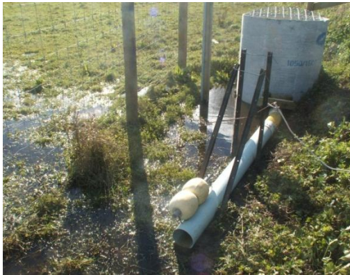
Figure 2.4: Floating decant structure after draining ponded water at Waiteti DB, May 2012.
