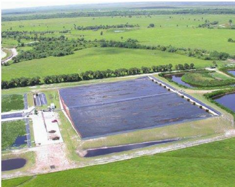
Figure 1.4: A large-scale ATS treating up to 1 million gallons per day of agricultural drainage water operated by HydroMentia, Inc near Lake Okeechobee, in central Florida (after Adey et al., 2011)
