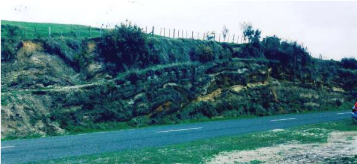
Photo of View Rd section taken in 2000 showing lower and upper parts
