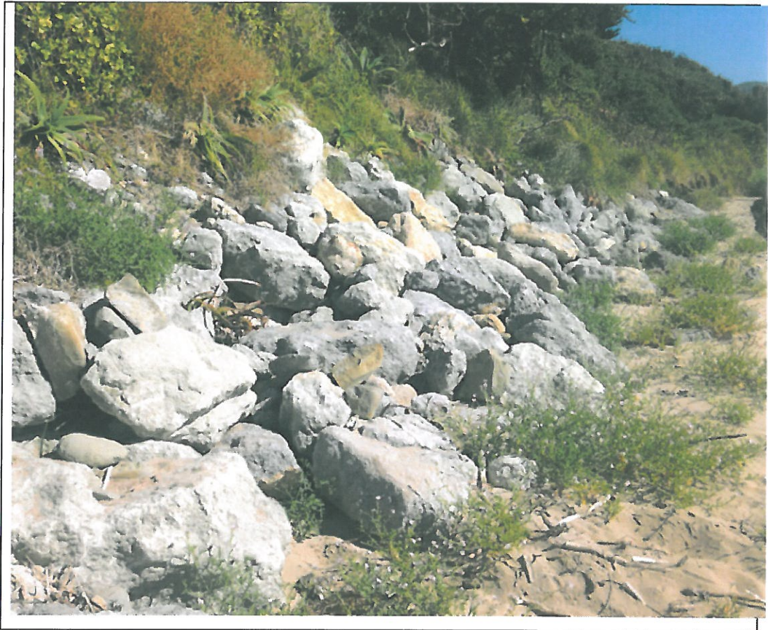
Figure 1- Rock revetment on Wainui Beach comprised of locally sourced boulders, which are degrading due to wetting and drying in a supra-littoral environment.
