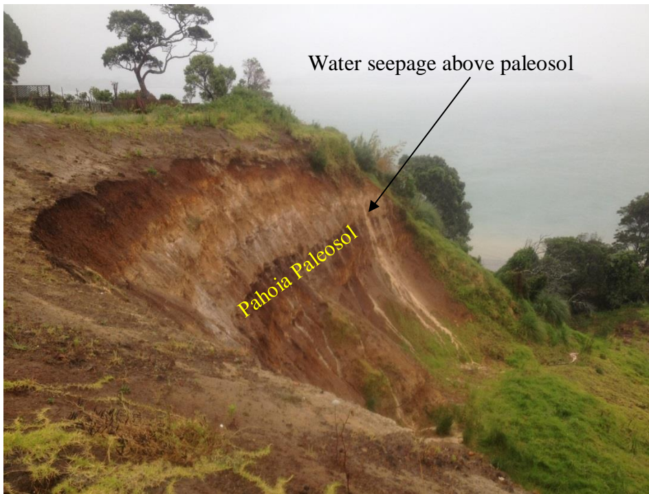
Figure 7.6: Water seepage above Pahoia paleosol layer at Bramley Drive (source: de Lange 2014)
