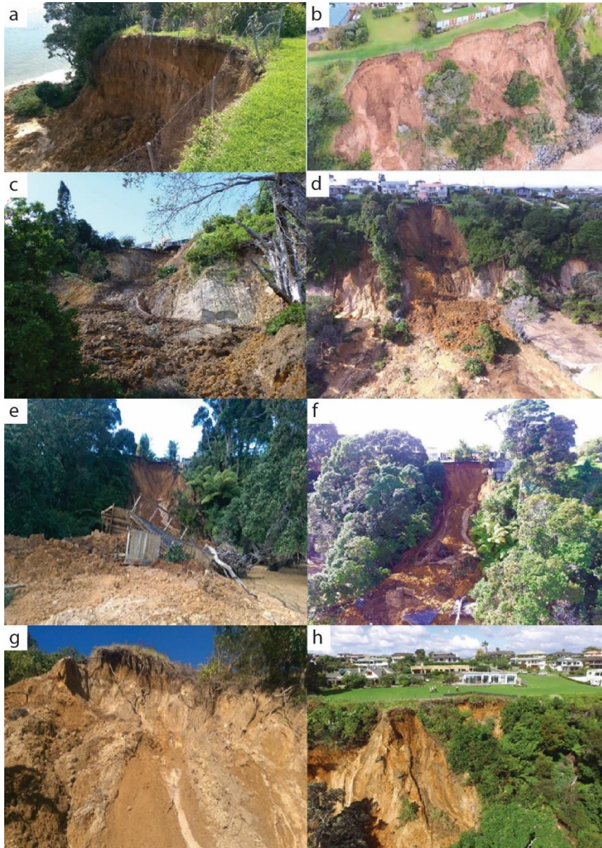
Figure 3.4(a) An aerial image of the Ruamoana Place landslide following the 2017 cyclone events within Ōmokoroa (as supplied by the WBoP District Council). (b) The same Ruamoana Place landslide was taken from the ground near the landslide scarp a few weeks after the landslide event. (c) The McDonnell Street landslide, as seen from the beach below, which failed a few days after the primary cyclone event. (d) Aerial drone imagery of the McDonnell Street landslide taken within 24 hours of the mass wasting event. (e) The Kowhai Grove landslide, as seen from the beach below the landslide a few days after the event had occurred; note the semi-intact deck carried down by the landslide debris. (f) The Kowhai Grove landslide photo was taken from aerial drone imagery soon after the landslide. Note the large amount of visible water exuding from the landslide scarp (supplied by WBoP District Council). (g) The Waterview Terrace landslide as seen from the beach below the landslide scarp. (h) The same landslide scarp at the Waterview Terrace taken from above via drone imagery (supplied by the WBoP District Council).
