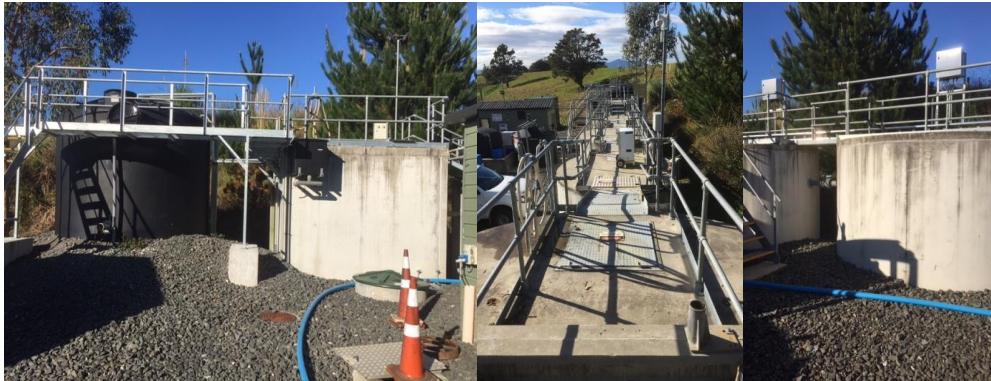
Figure 11. Photos were taken at Tahuna treatment plant showing the treatment tanks
