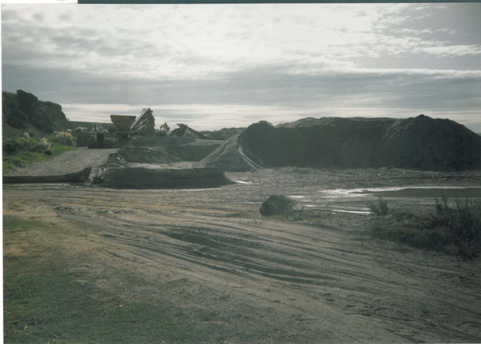
Figure 2.10a & b Sand extraction at Otamarakau, where sand is mined from between the berm and dune. This activity over 35 years has resulted in complete decapitation of the dune and only dune ridge. Figure a) shows the site in April 1992, and b), a year later in April 1993 with a noticeable stockpiling of sand estimated at 12,000 m 3 or 90% of the operators annual limit (Brett O'Shaunessy pers. comm. )
