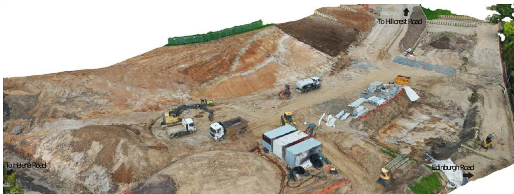
Figure 4.2 Still from drone footage of the site at 59 Hillcrest Road, Hamilton. Viewing toward east-northeast.
