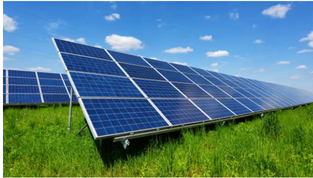
Figure 2-14: Solar power field [9]
