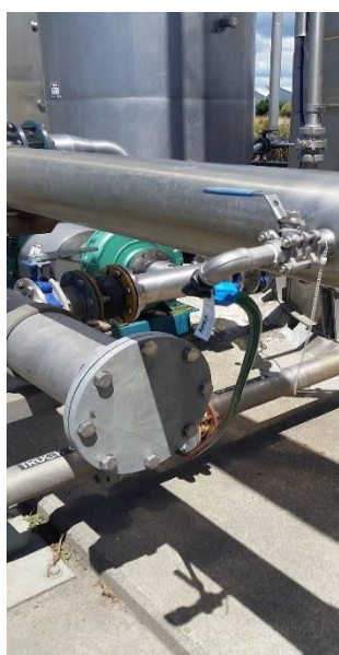
Figure 3-10. Hose connected to Awakeri effluent line.
