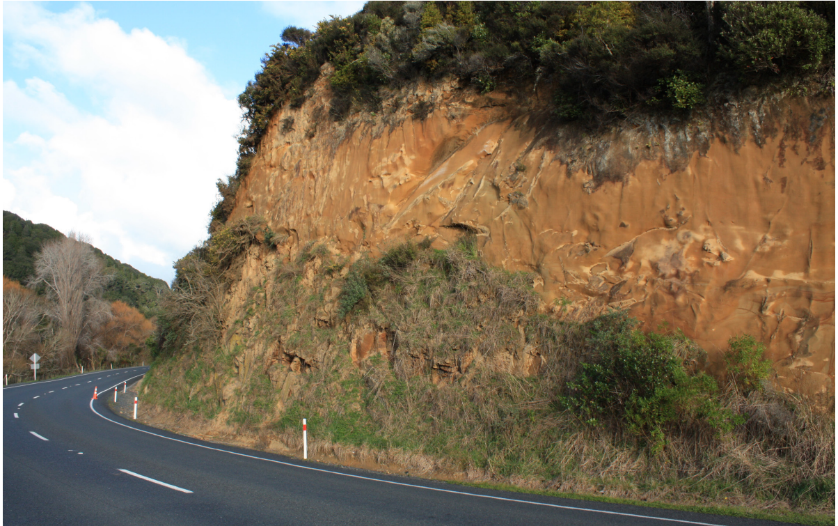
Fig. 24A. Rusty brown weathered Bexley Sandstone (Pl) on irregular relief (top of grassed face) on late Triassic Murihiku terrane basement at the SW end of Awakino Gorge.
