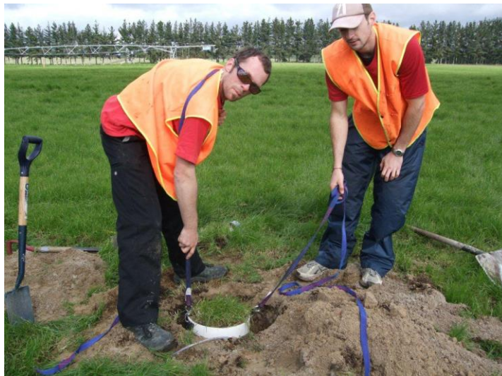
Figure 3.6. Installation of lysimeter within the field. Photo, Glen Treweek.
