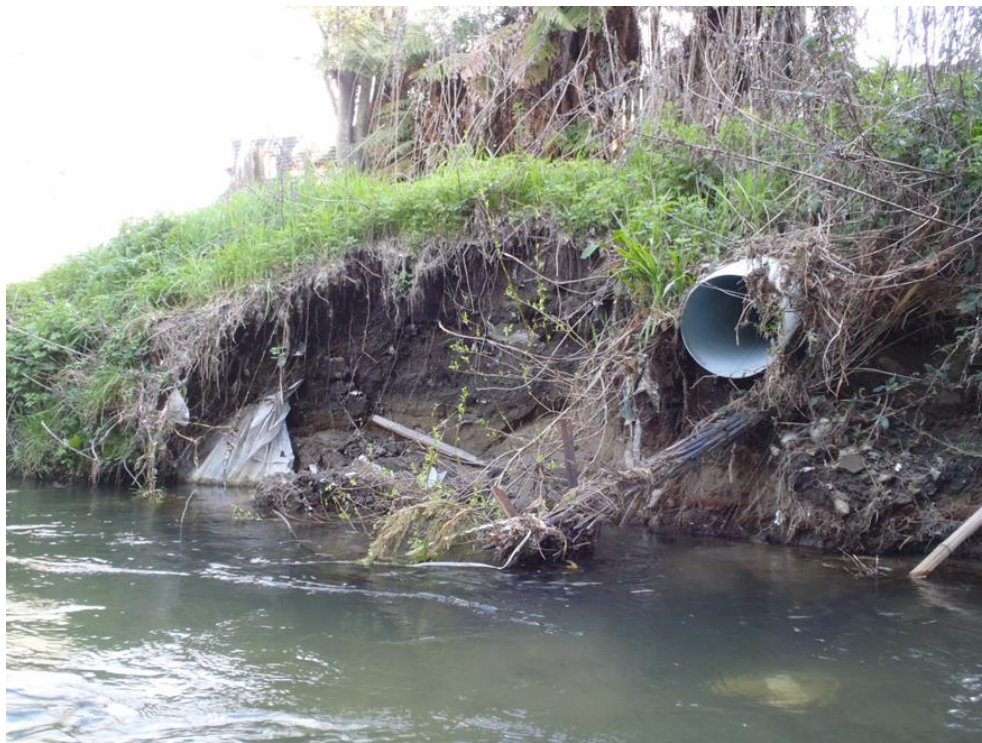
Figure 9. A stormwater drain (Site 1 true right bank) installed without adequate bank reinforcement (From: Ling, 2013).
