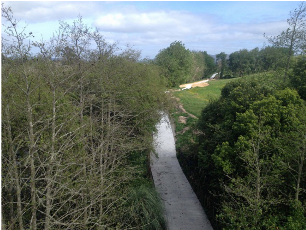
Figure 9. Te Awa River Ride, construction of the Horotiu-Ngāruawāhia section during spring 2017. Source Rodrigo Hill 2018.
