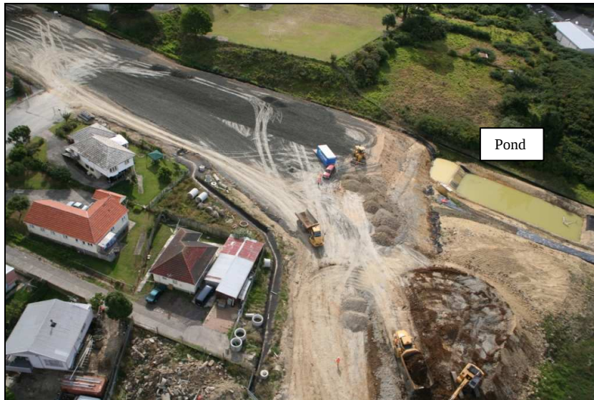
Fig. 5.20: Aerial view of the Richardson Road pond on 09/03/07. The site is being actively worked, and the high turbidity levels in the pond are evidence of sediment laden runoff (Photo courtesy of Transit, 2007).
