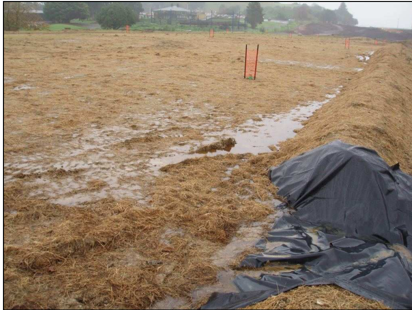
Fig. 2.3: Water ponding on a compacted surface.
