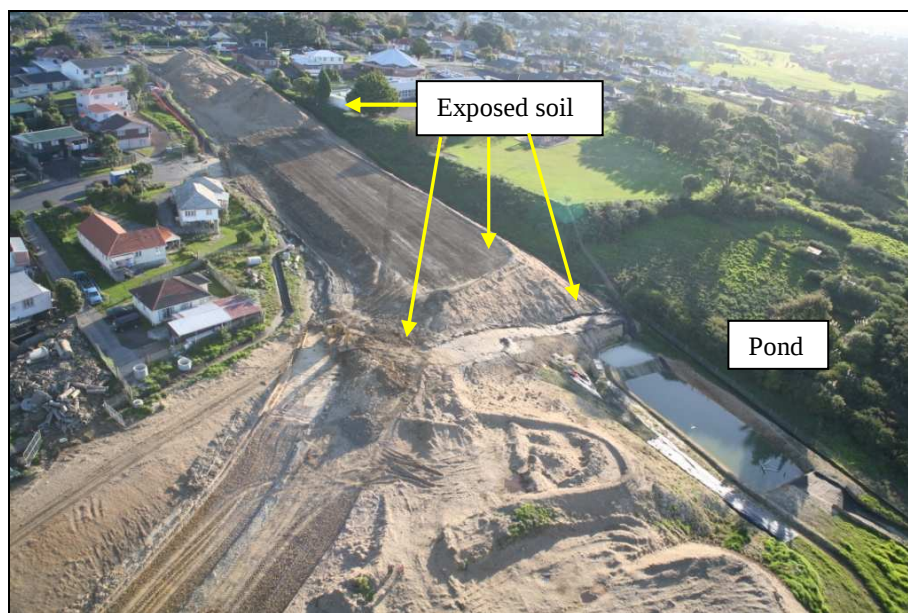
Fig. 5.23: Large areas of unstabilised soil upslope of the Richardson Road pond on 07/05/08 (Photo courtesy of Transit, 2007).
