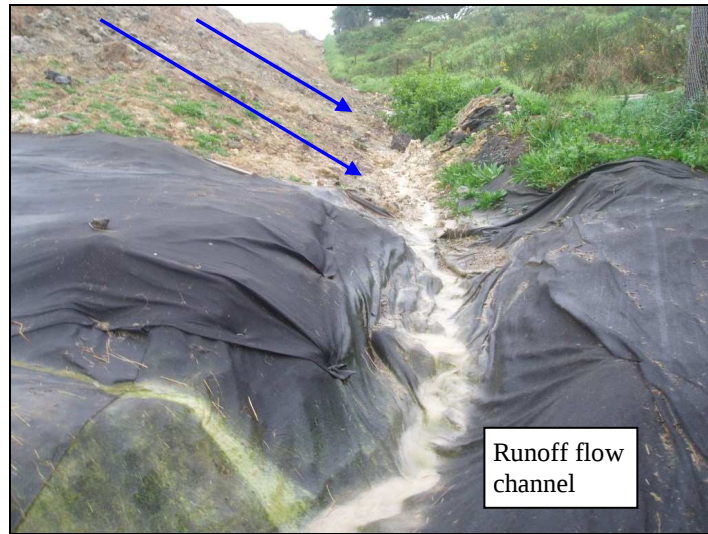
Fig. 6.9: Exposed soil and high runoff velocities meant that increased sediment reached the Richardson Road pond.
