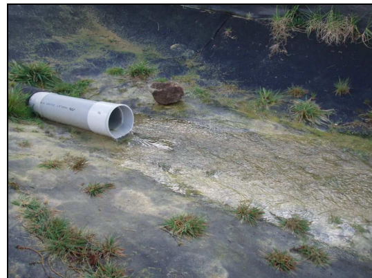
Fig. 5.27b: The extended discharge pipe on 15/05/07.
