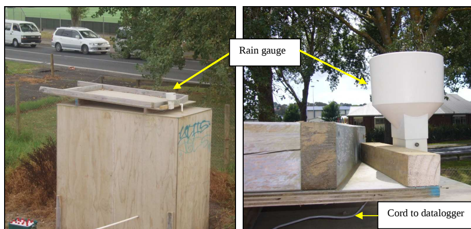
Fig. 4.7: Rain Gauge installed on the roof of the chemical dosing shed at Somerset Road pond.
