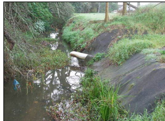
Fig. 3.12b: Discharge pipe above the Oakley Creek Tributary
