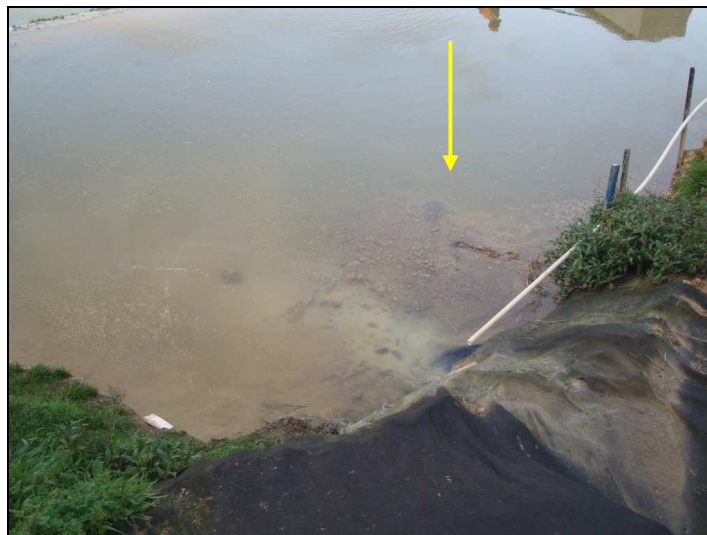
Fig. 6.10: Development of a sediment delta at the entrance to the Richardson Road forebay on 17/07/07.
