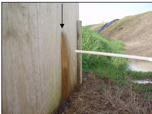
Fig. 6.3a: Pipe disconnected from the side of the chemical dosing shed on 12/08/07.
