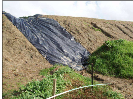
Fig. 3.11b: Stabilised inlet to the Somerset Road pond, July 2007.
