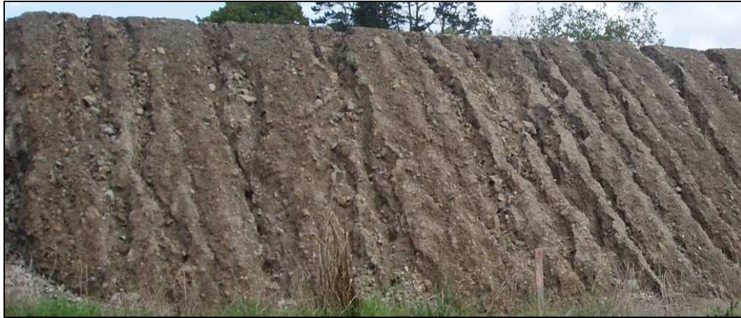
Fig. 2.2: Gully erosion on a bank.
