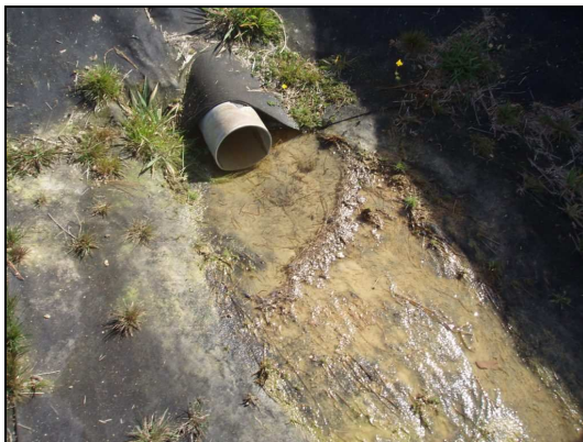
Fig. 5.27a: Accumulation of algae on the geotextile mat below the Richardson Road discharge pipe (02/04/07).
