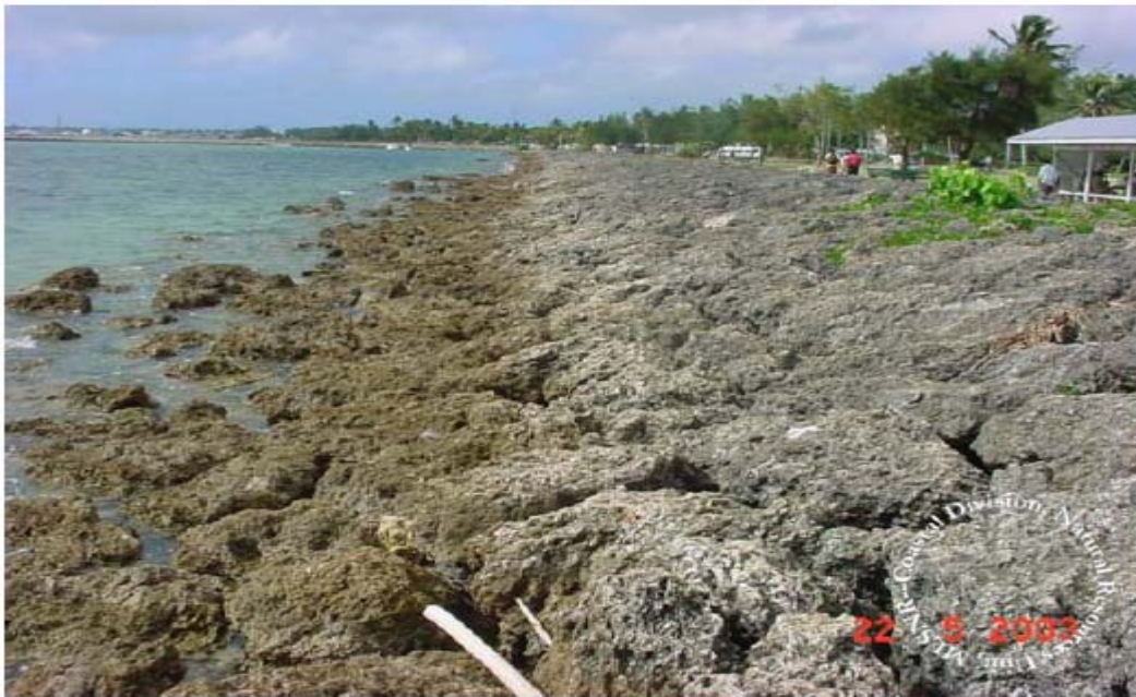
Figure 2.18: Coastal Foreshore Protection Wall at Nukuálofa Waterfront Source: Ministry of Lands, Survey & Natural Resources, 2003.
