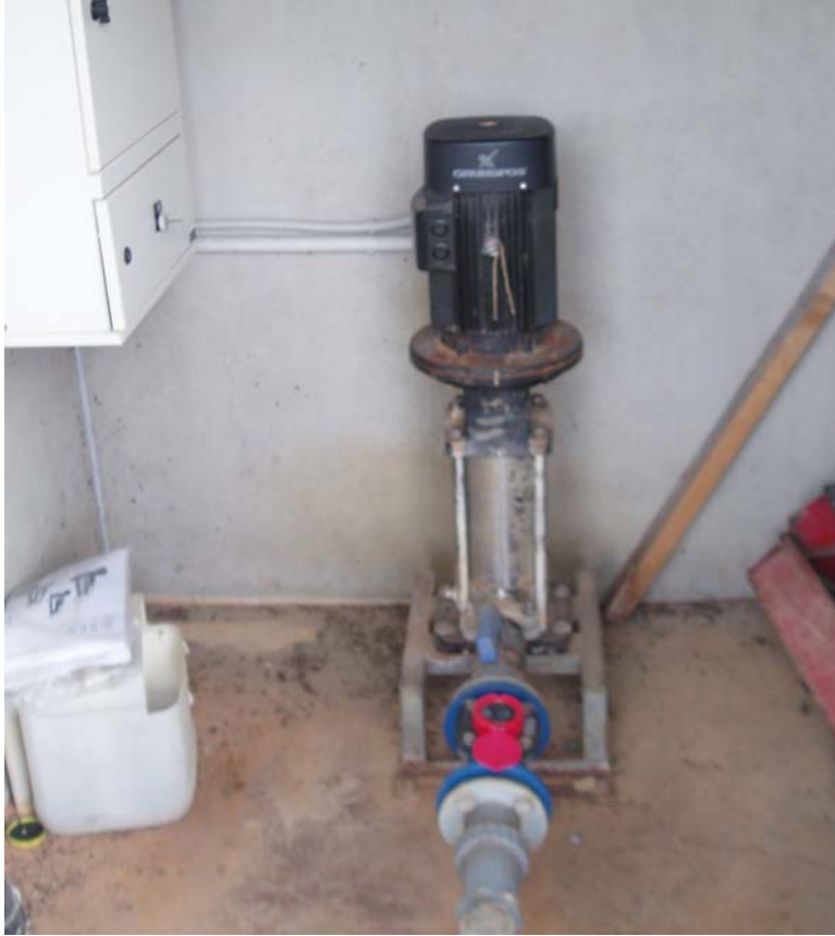
Figure 3.12: Leachate Irrigation Pump.
