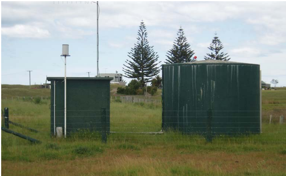
Figure 3.10: Leachate collection tank and pump house.
