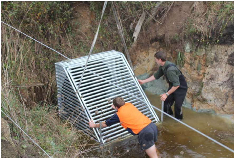
Figure 7. Adam Daniel and Daniel Hall installing the adult pest fish barrier in the Lake Ohinewai drain on the north side of the Tahuna Road culvert 5 May 2011. Photo: A. Gray.
