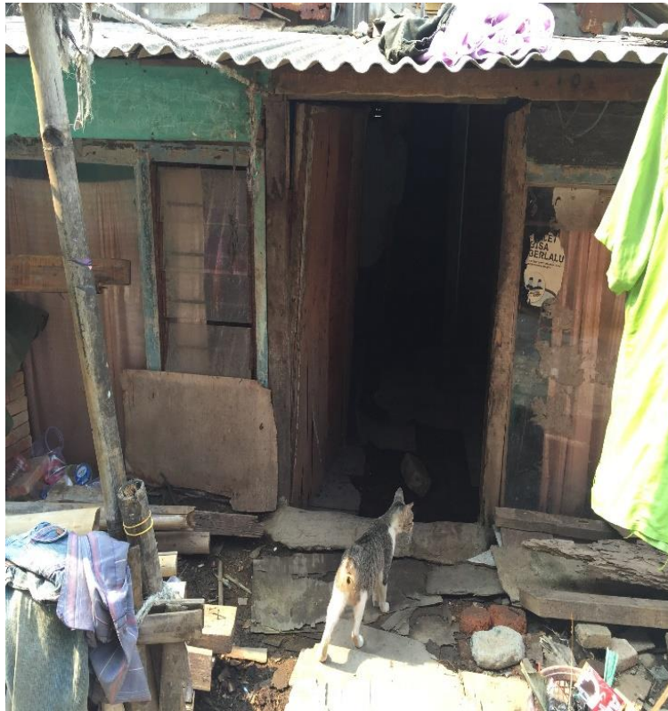
Figure 11 Joko's house which is lower than the walking path in front of his house. (Source: Author).
