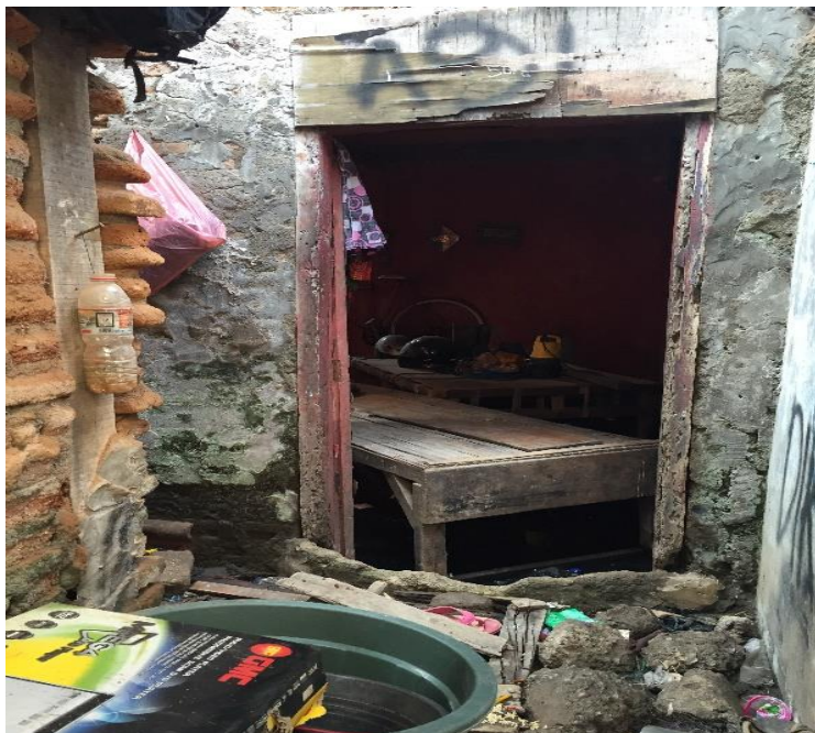
Figure 13 First floor of a house was abandoned due to frequent flooding events. (Source: Author)
