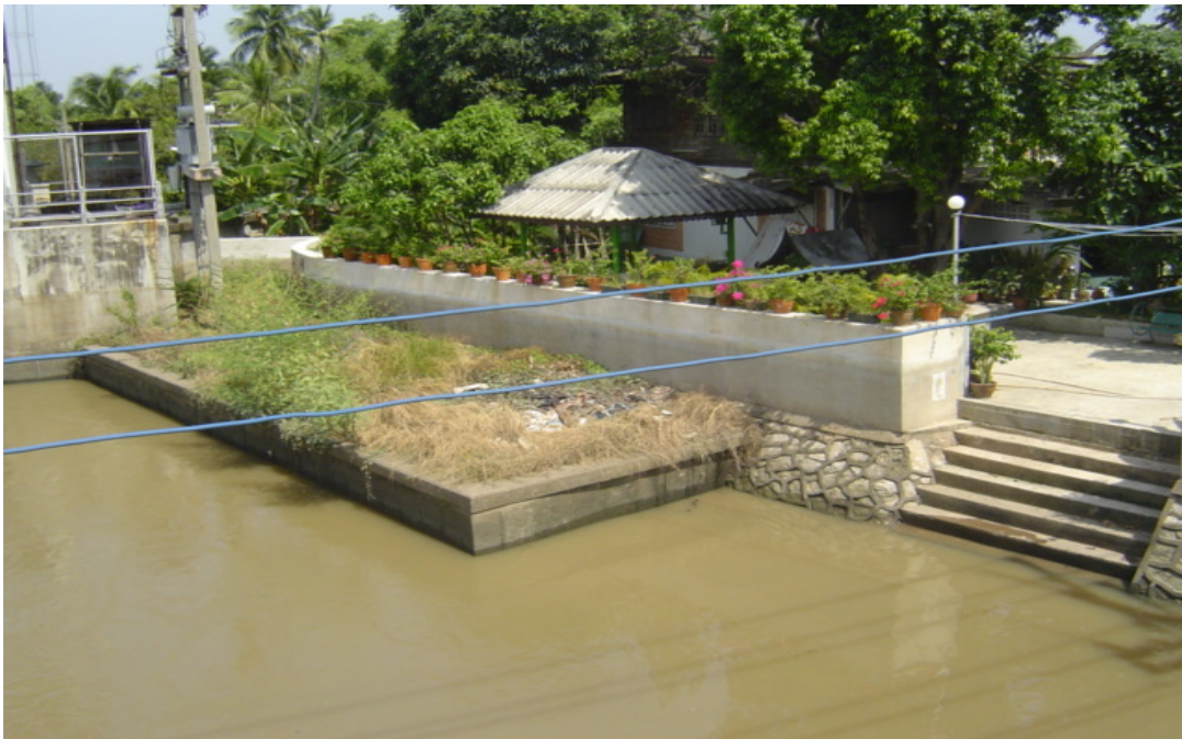
Figure 15 Concrete wall built by the homeowner (Washaree), Note: The lighter colour showing the water mark and the increased height of the wall.
